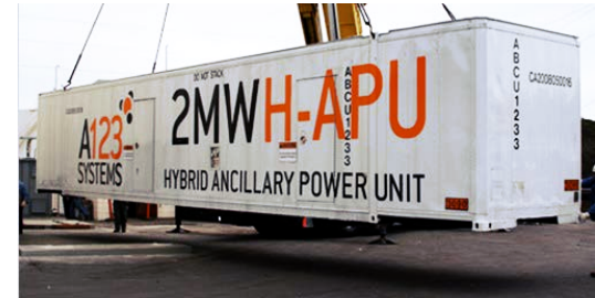
Large Scale Stationary storage (utilities)
